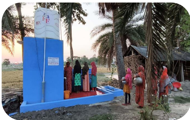
Submersible Water Pump at Gangachori Khalpar, WB
