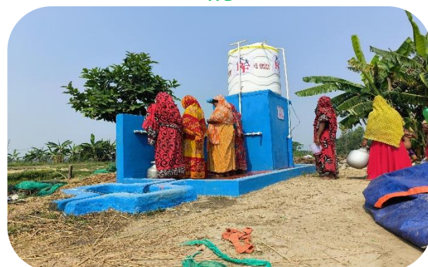
Submersible Water Pump at Hamidpur, WB
