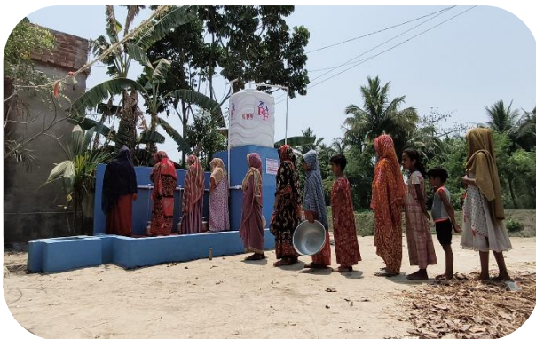
Submersible Water Pump at Sarangabad, WB
